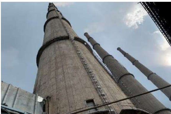
Project site of Condition Assessment of RCC Chimneys of Kolaghat Thermal Power Station, West Bengal PDCL.
