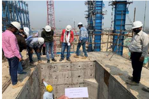
UPV Test on TG Deck Slab at a power plant project site in Uttar Pradesh
