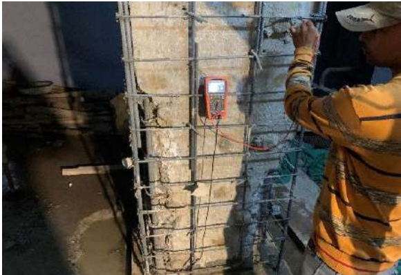
Continuity testing being done after installation of Zinc anodes at site of NHAI Residential Enclave at Dwarka, New Delhi
