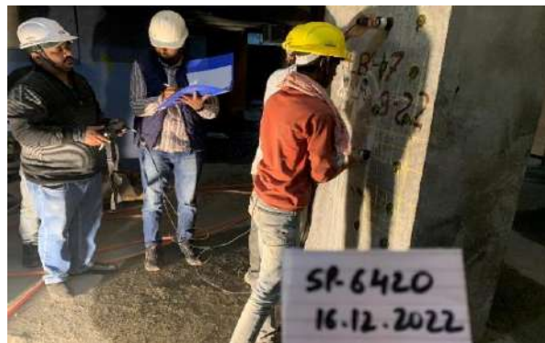
Random Quality Inspection during repair at NHAI Residential Enclave at Dwarka, New Delhi
