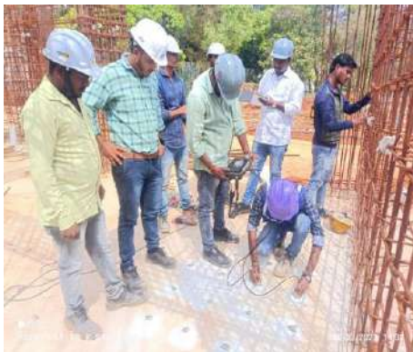
NDT Work of Construction of Additional Infrastructure at IISc Main campus, Bangalore
