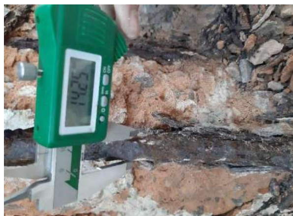
Measurement of existing rebar diameter of an RCC member at a Building site in Delhi
