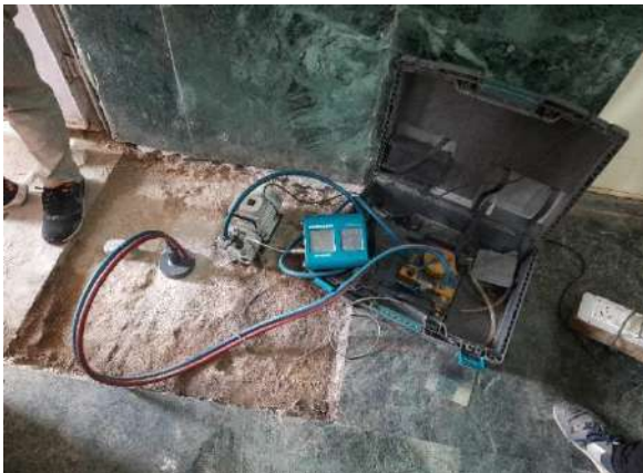
Air Permeability Test on the slab of a building structure in Delhi
