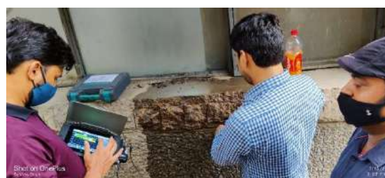
Measurement of Half-Cell Potentials of reinforcement on an identified beam in NCB premises
